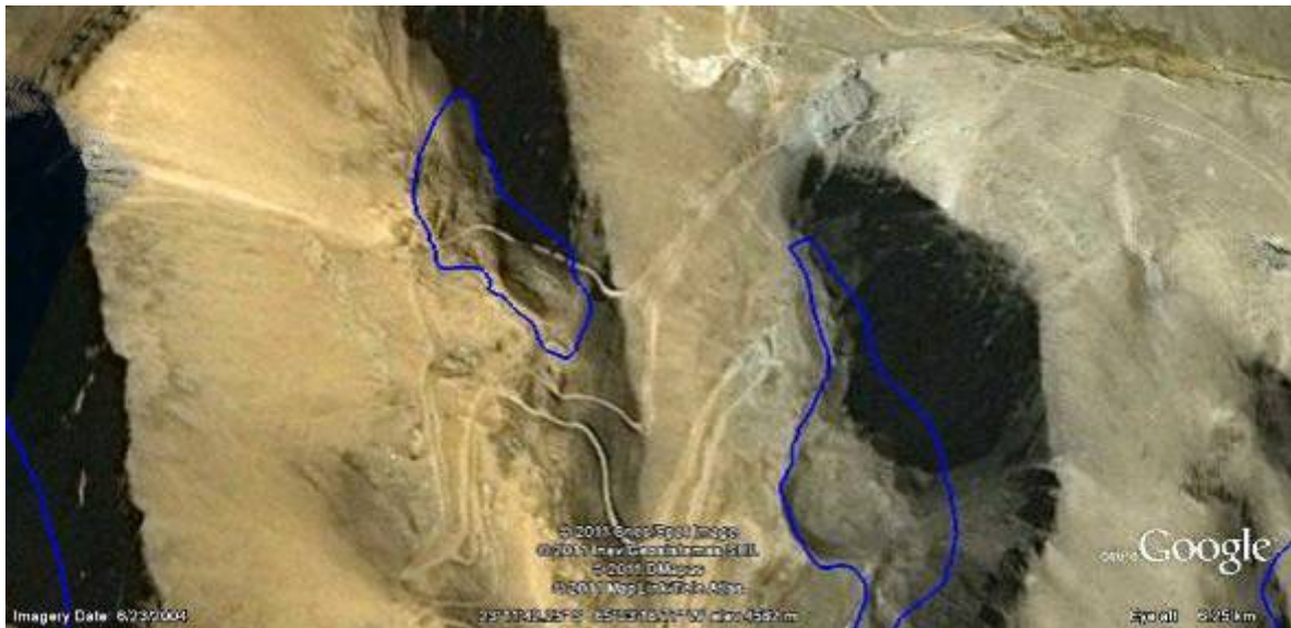
Road Works in border area of Jujuy and Salta cross rock glaciers and impact periglacial environments.
